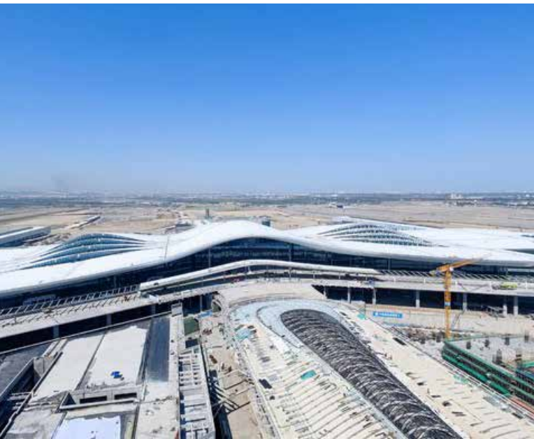
The Urumqi Diwopu International Airport, which is undergoing reconstruction and expansion, in Urumqi, northwest China's Xinjiang Uygur Autonomous Region.
